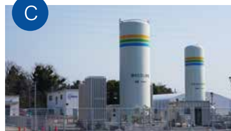
CO 2 supply equipment
